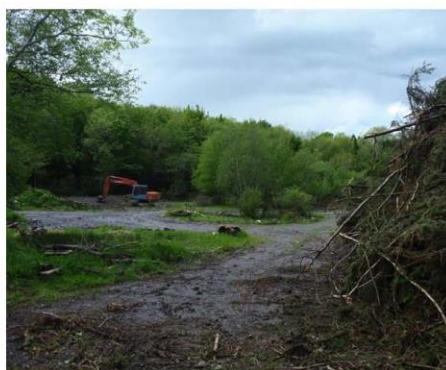
Photo 1.4: Infilling of site, to the south of the N16 (view to west)
